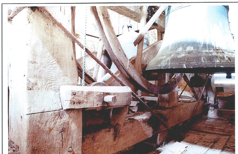
Fig. 16: The bell frame, centre pit, north truss. A Lester & Pack 1754 bell in foreground
